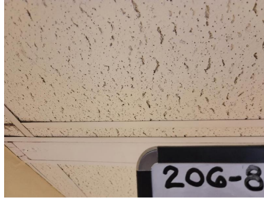
206-8 2'x4' Suspended Ceiling Tile Typical Interior
