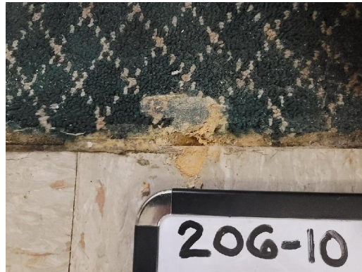
206-10 Carpet Mastic Typical Interior
