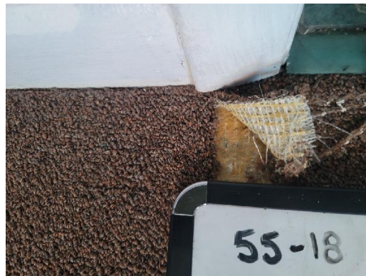
55-18 Carpet Mastic Typical Interior
