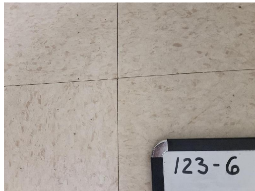
123-6 12"x12" Floor Tile/Adhesive Interior Front Entry
